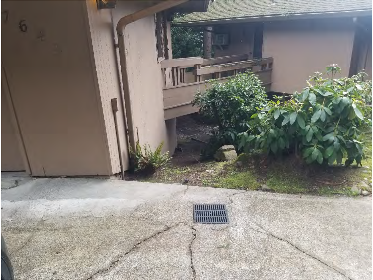
Surface Inlet to Pipeline at Corner of Garage, Pipeline Runs Downhill Under Wood Bridge
