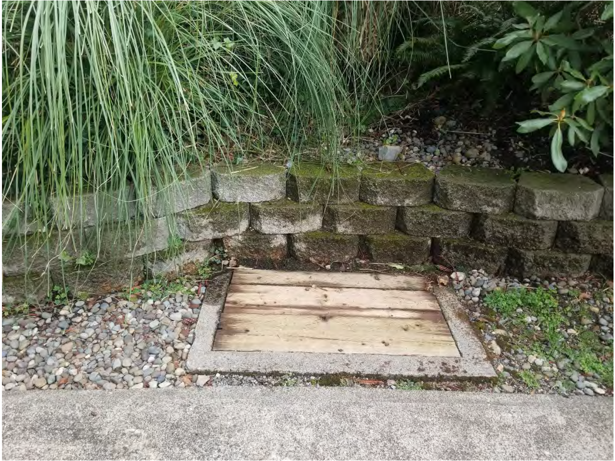
Wood Lid Pipeline Box
